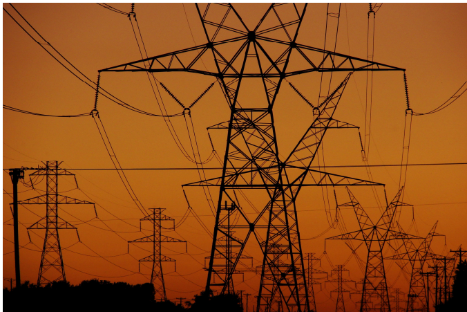
Figure: Power lines
